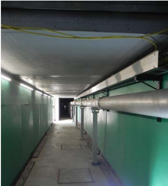
FP13 Beam line, downstream
